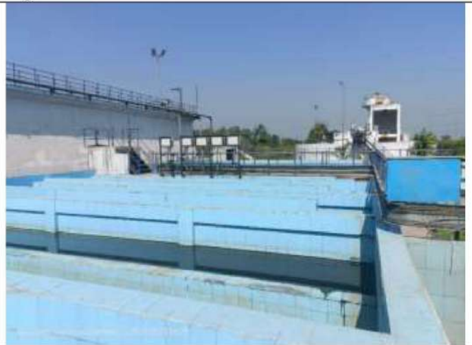
Fig 4: Chlorine contact tank
