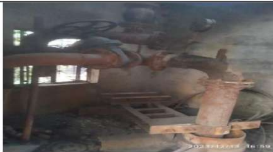
Photo 15: Borewell in distillery plant
