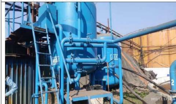
Pic.-13.Sludge drying bed
