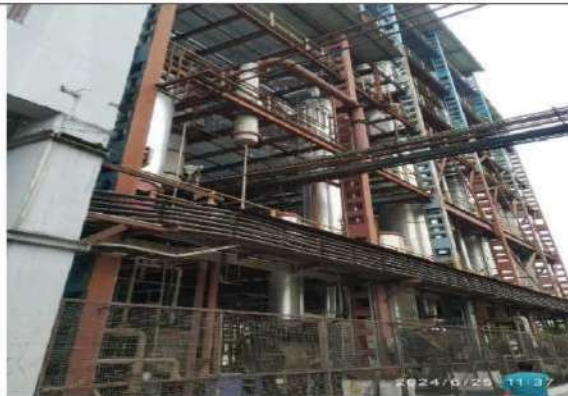
Photo 6: Distillery machineries non-operational
