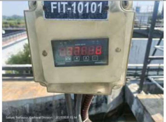
Fig 2: Inlet flow meter
