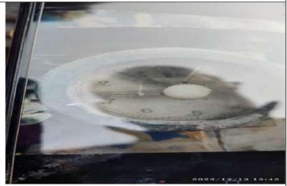
Pic.-20.Leakages in fresh water pipeline
