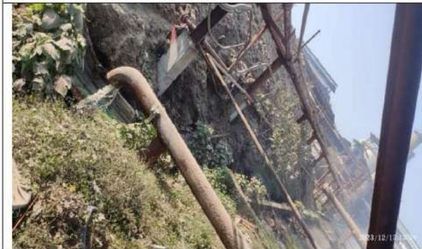
Pic.-17.Flow meter at inlet of SRS
