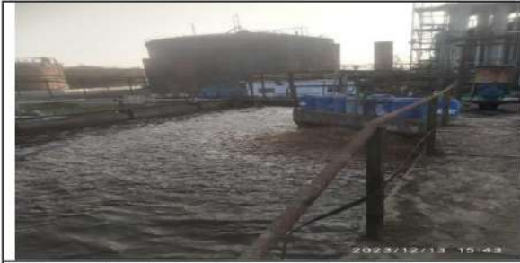
Photo 11: Aeration tank in CPU
