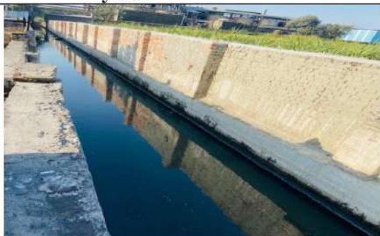
Photo 19: Laksar drain passing from the premises
