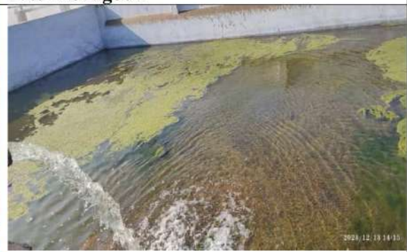
Pic.-14.Spray pond overflow treatment unit
