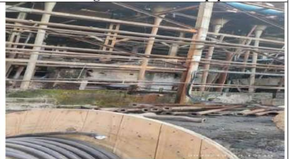
Pic.-22.Clear juice heater on computer system
