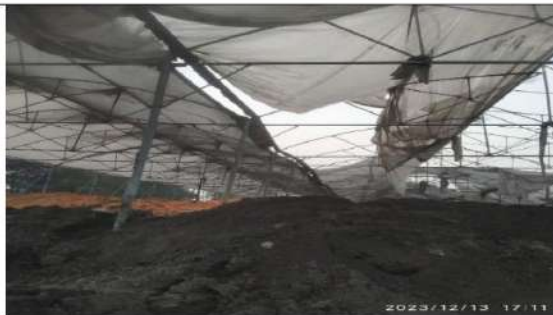
Photo 17: Damaged shed in bio-compost yard
