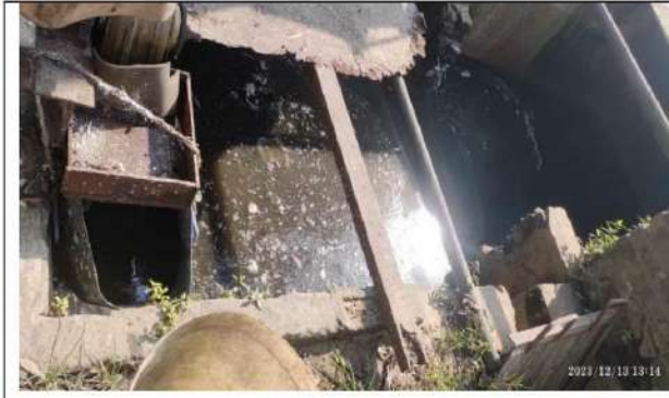
Pic.-07.Equalization tank without air mixing arrangement
