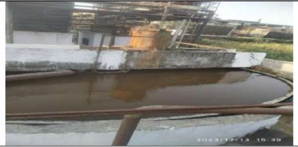
Photo 12: Secondary clarifier in CPU
