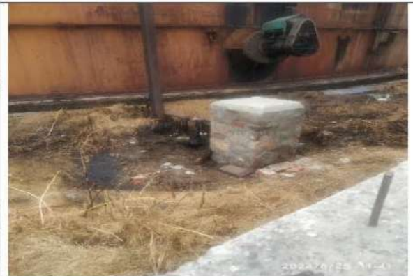
Photo 7: Distillery Piezowell found sealed with concrete
